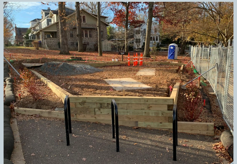
The new bike racks have been placed. The timber edging is being installed and some rough grading of the site along with perimeter plantings has begun.
