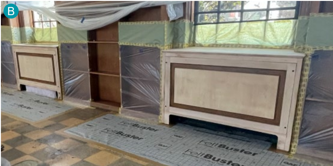
Existing wood elements along perimeter being hand sanded and will be refinished.
