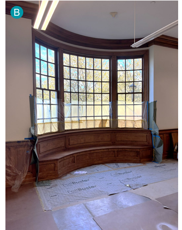
Progress in April: Refinishing of the wooden bench and lighting installation is complete.
