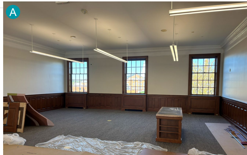
Progress in April: carpet, floor boxes, and lighting installation is complete. Wall painting, build out of the service desk, and selective wood refinishing in progress.
