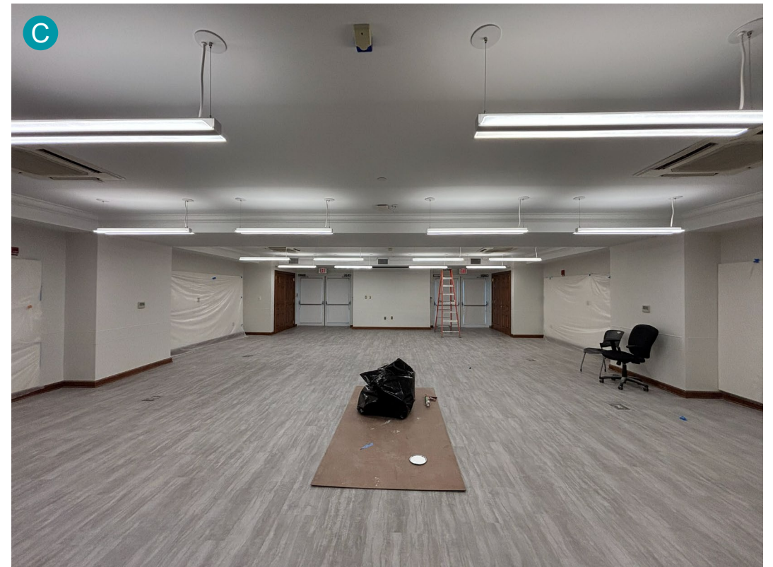
Installation of LVT and lighting is complete in the Meeting Room. Wall painting is in progress.
