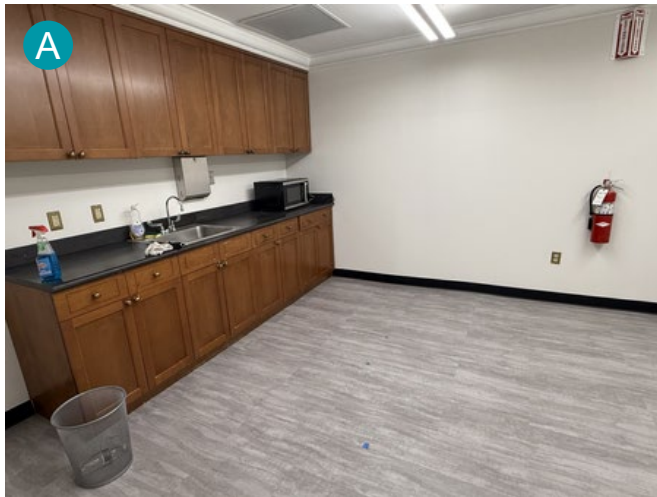
Installation of flooring and new lights and wall painting is complete in the Staff Lounge.
