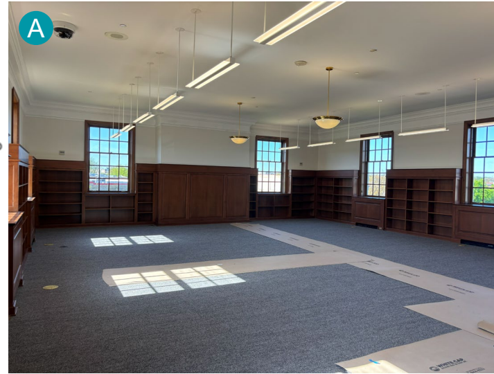
Progress in April: carpet, floor boxes, and lighting installation is complete. Wall painting and selective wood refinishing are in progress.
