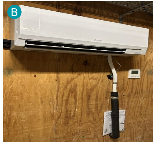
Installation of the new air conditioning unit in the IT Room is complete.
