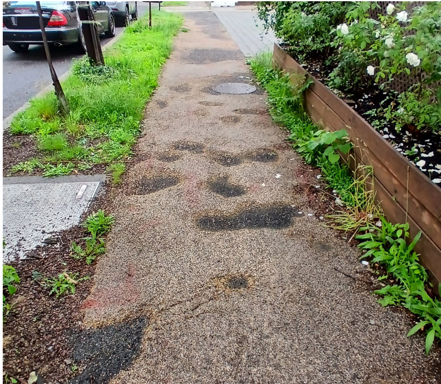
There were several locations in the school zone where the sidewalk was cracked or heaved. The example shown in the image above with severely deteriorated flexible pavement is on Webster St near the school.
