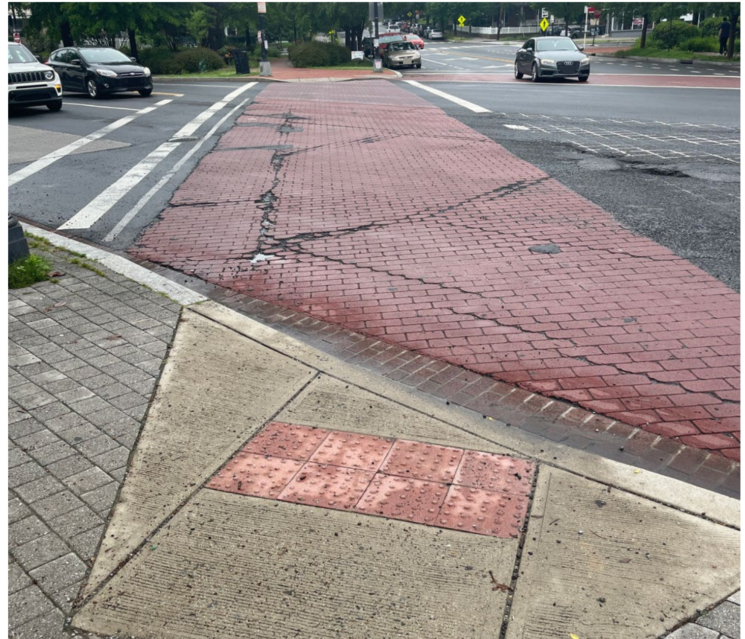
The crosswalk markings at the intersection of Georgia Ave and Kansas Ave are not highly visible. The north crosswalk across Georgia Ave is in poor condition with multiple holes, cracks, seams, and ripples in the surface.
